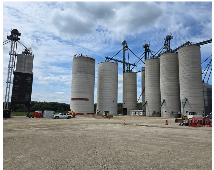
Pictured: Expansion at our Drayton, ON location, includes two new concrete silos, that were completed in time for the 2024 harvest.
